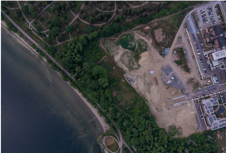
This shot was captured by drone on June 6, 2021. Builders have excavated and regraded the sandy soil all the way up to the eastern boundary of my observation site, laying the groundwork for several new apartment buildings and a hotel.
